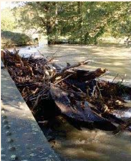
Figure 41 Debris washed up against a metal bridge deck
