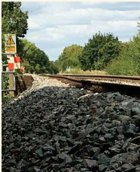
Figure 23 Image showing track alignment issues when transitioning to underbridge
