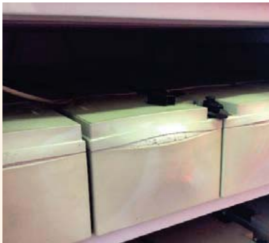
Figure 24 Overheated batteries, Southall UPS, August 2015
