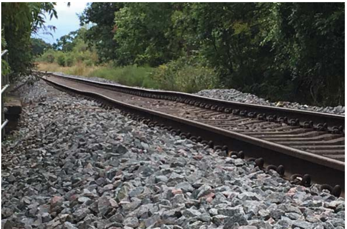
Figure 33 Poor track geometry due to heat impact
