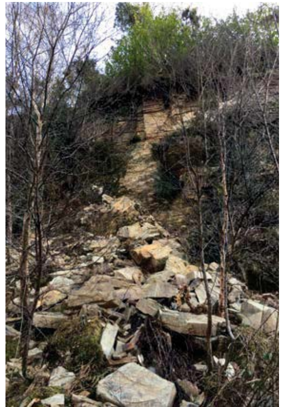
Figure 30 Rockfall failure occurring on MLN3 in 2018
