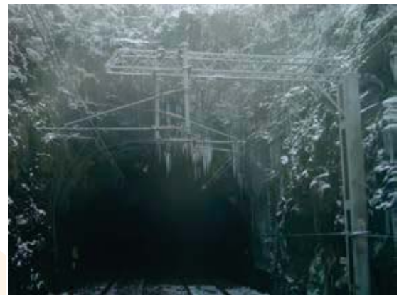
Figure 36 Icicles formed around OLE equipment, (note –picture not on Western Route)
