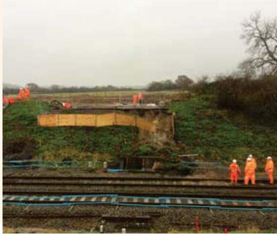
Figure 29 Washout failure and adjacent field at Chipping Sodbury Aqueduct (SWB 103m 74ch Dn)
